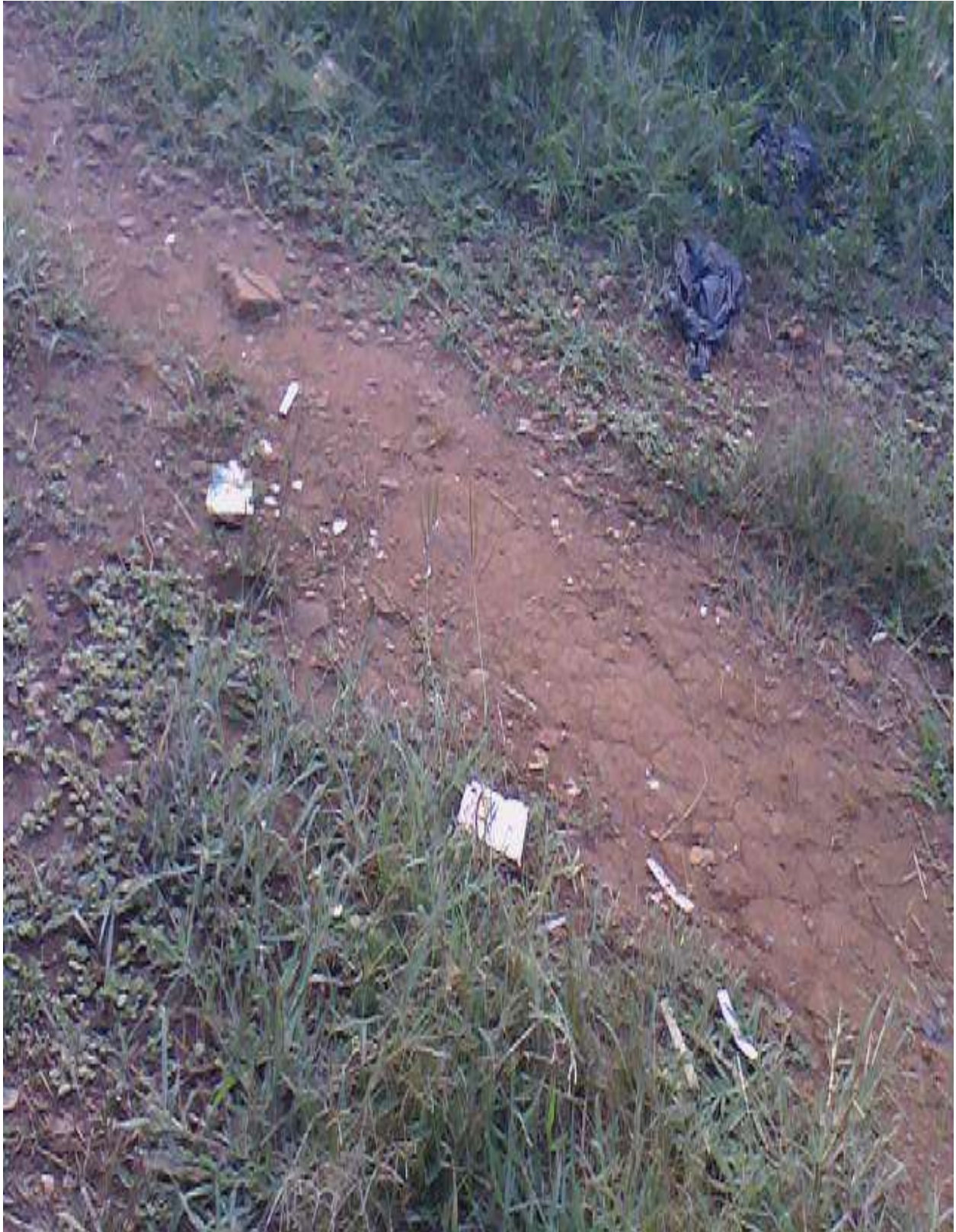
FIGURE 6: A photo showing roads in a poor condition.
