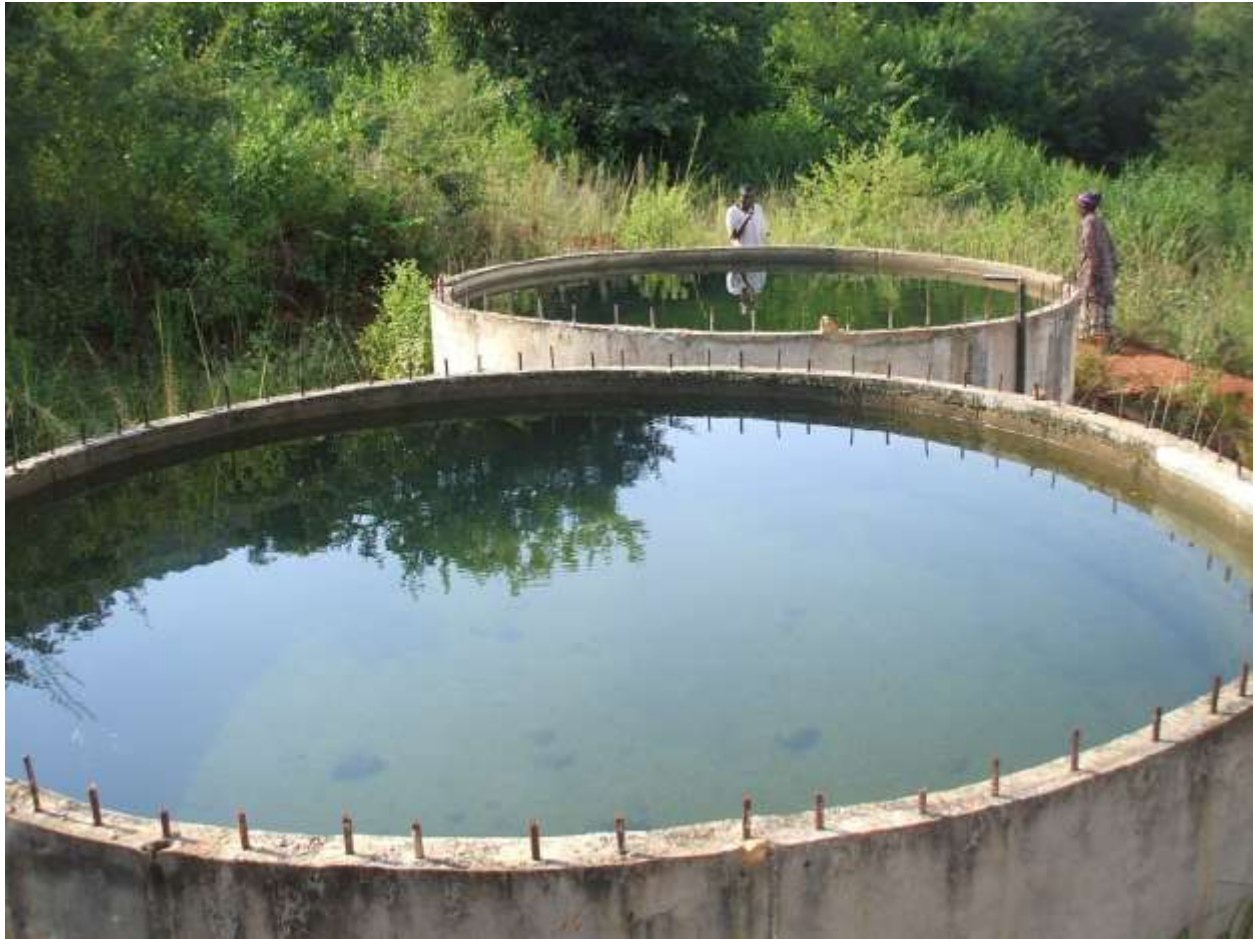
FIGURE 4: A photo showing unsafe water reservoir that provides water to the project and the tap to the community.
