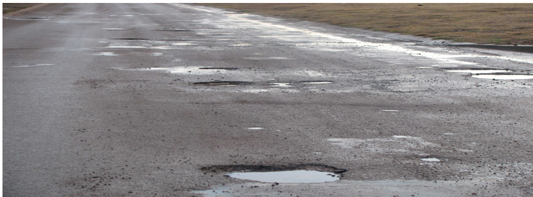
Figure 2. Potholes in Sharpeville
