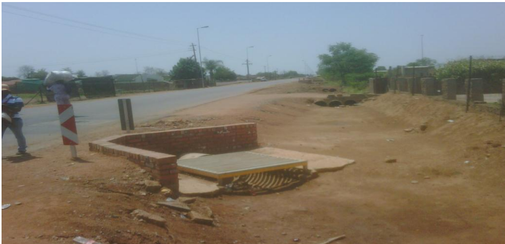
Figure 10: A newly constructed roads and stormwater drainage in Soshanguve (North West Region of CoT)
