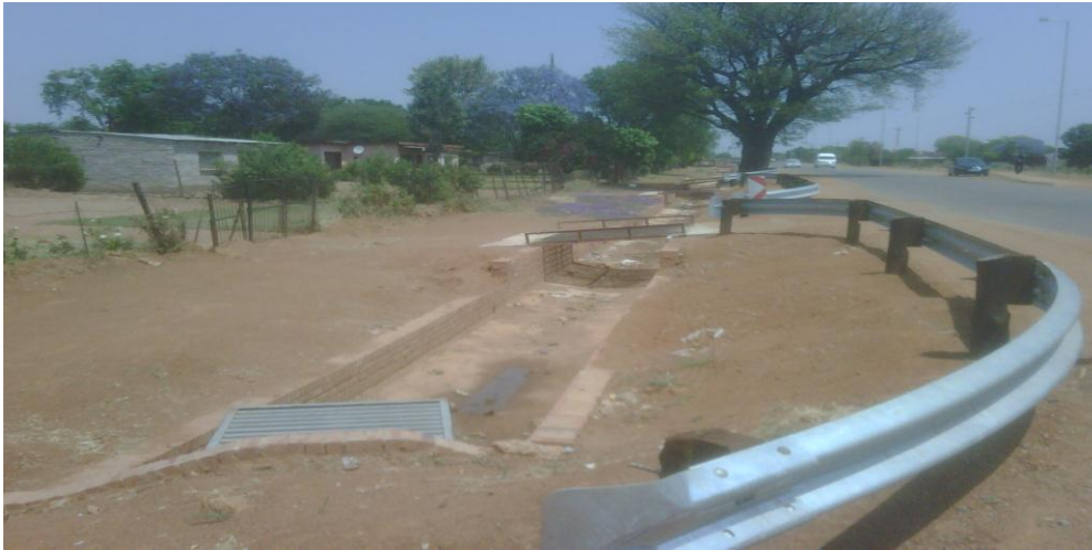
Figure 9: A newly constructed road and stormwater drainage in Themba Community (North East Region)
