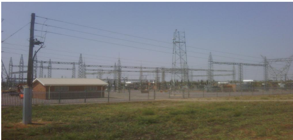
Figure 5: Themba Electricity Sub-station reticulating to population (North East Region).
