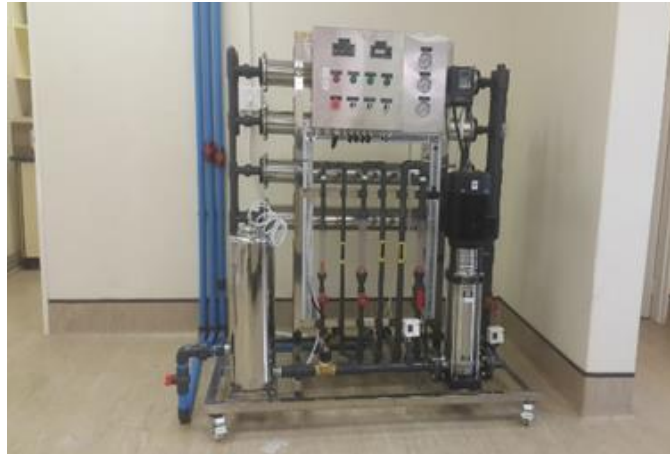
Figure 1.4 2.4 m 3 /h RO stage of the R&D plant at the University of Limpopo (Commissioned in 2018)
