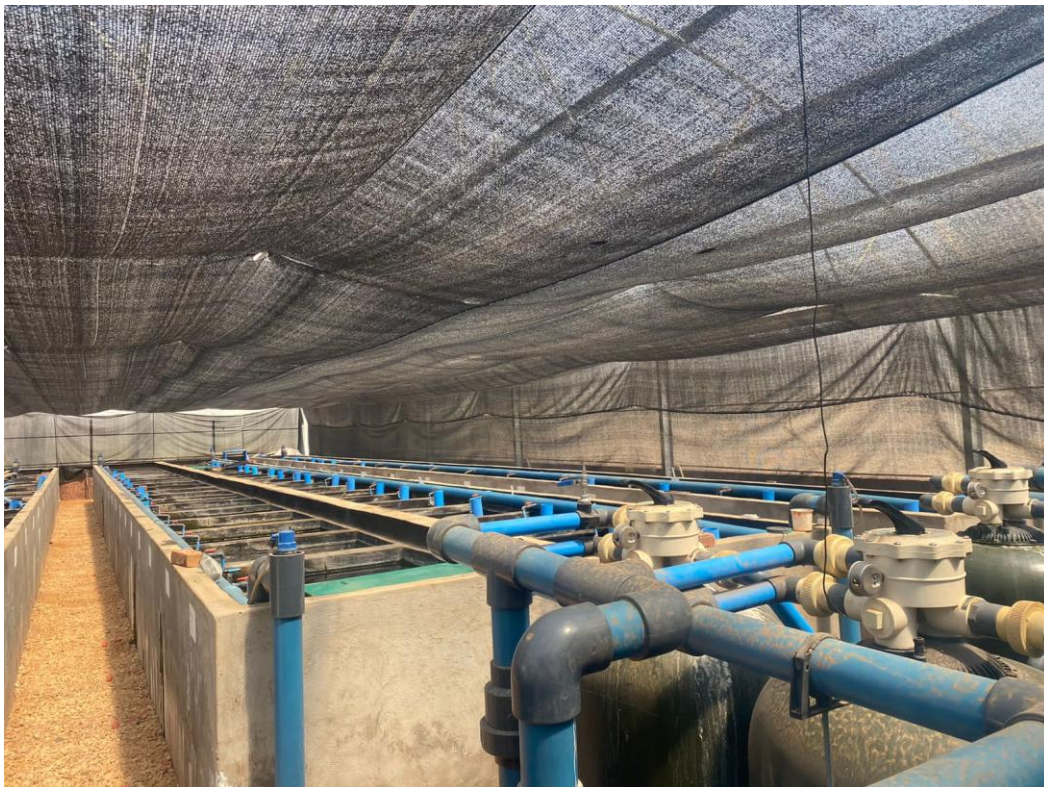
Figure 3. 1: The rectangular concrete tanks connected to a recirculating system at the Aquaculture Research Unit, University of Limpopo, South Africa.
